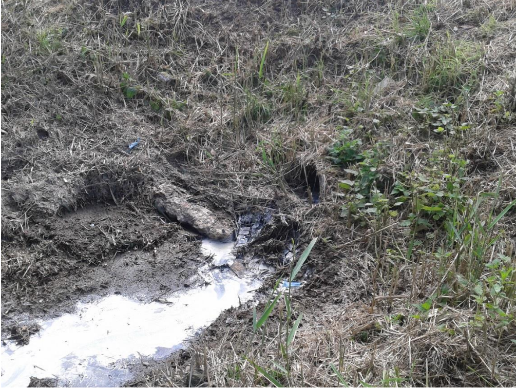
Plate 3: A partially collapsed culver outfall in Boston 4
